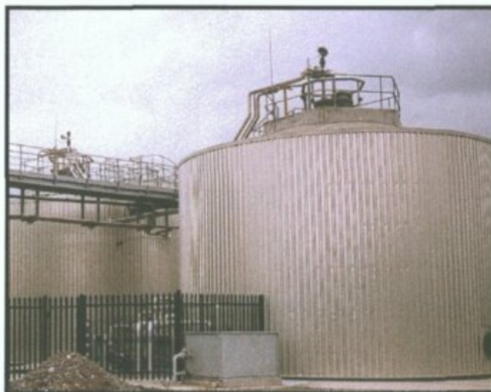
PLATE 3.5.3 CLONMEL ANAEROBIC DIGESTERS
