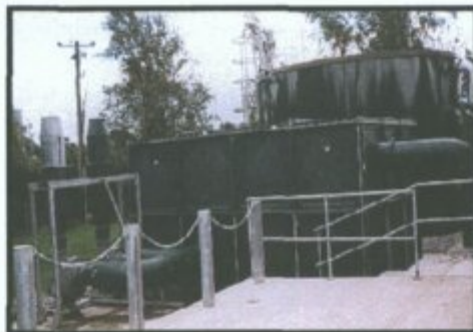
PLATE 3.2.8 ODOUR CONTROL SHELL FILTER
