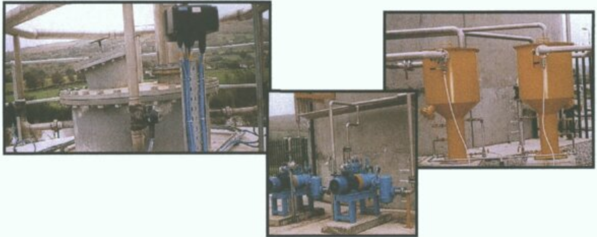
PLATE 3.5.5 GAS DROP PIPES ENTERING AT THE TOP OF THE DIGESTER, GAS COMPRESSORS & GRAVEL FILTERS
