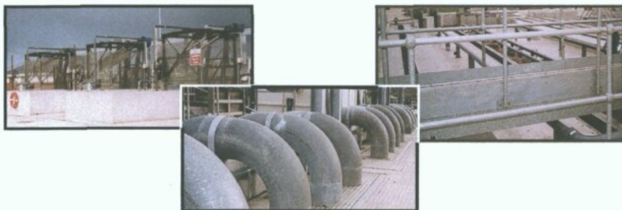
PLATE 3.5.1 INLET CHAMBERS, TOP OF SUBMERSIBLE PUMPS & HARTMAN TANK
