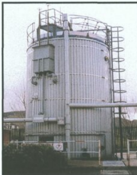
PLATE 3.3.3 BUNCRANA ANAEROBIC DIGESTER
