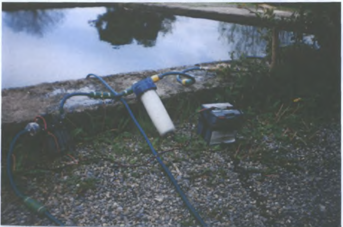
Fig. 3.2: Cryptosporidium rig in situ in Clonmel Water Treatment Plant. Picture shows from left to right: Pump, Cartridge housing, Battery, Flow restrictor and meter. Hose is in Raw Water sump.
