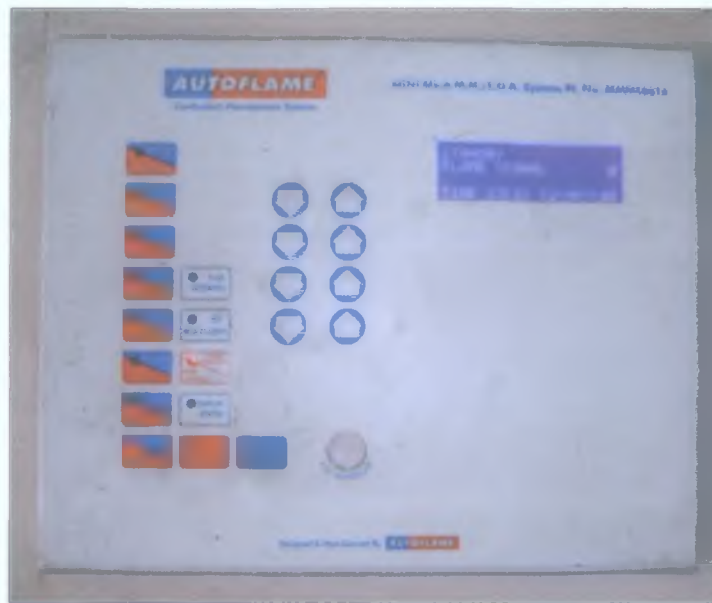
Plate 4.5.3 Autoflame Control Panel
