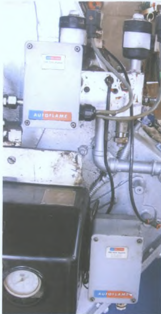
Plate 4.5.2 Autoflame conversion kit on the Beel boiler
