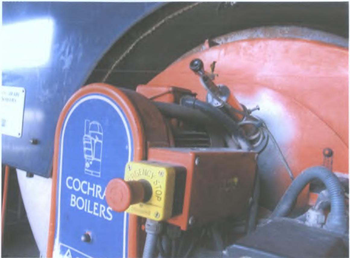
Plate 4.5.7 Infra-red temperature sensor on the Cochran boiler
