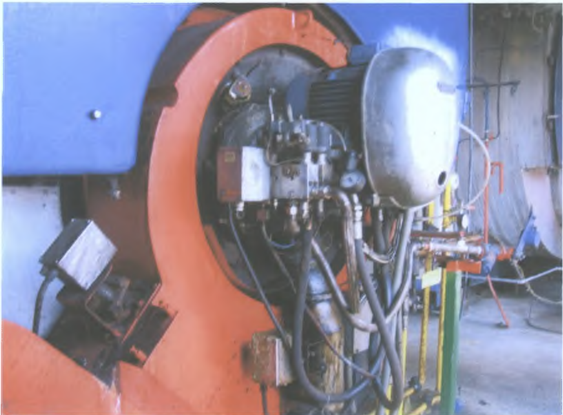
Plate 4.5.4 Autoflame conversion kit on the Ruston Boiler
