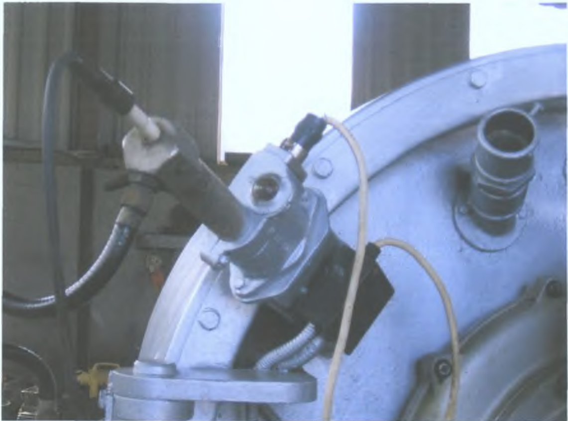
Plate 4.5.6 Cylindrical housing (on the far right) for the infra red temperature sensor on the Beel Burner.
