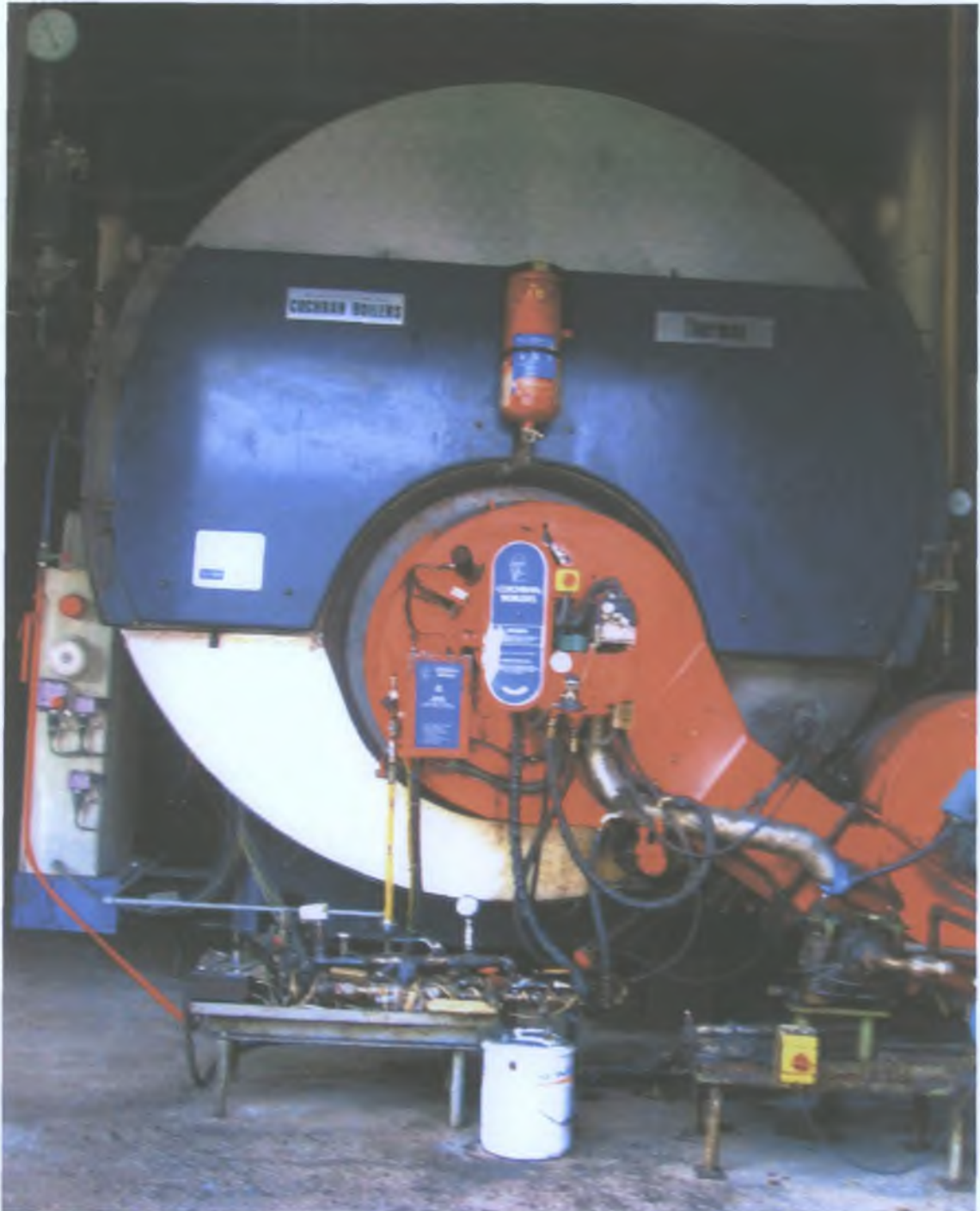
Plate 4.5.1 Cochran boiler with the tallow conversion kit at the base on the left.
