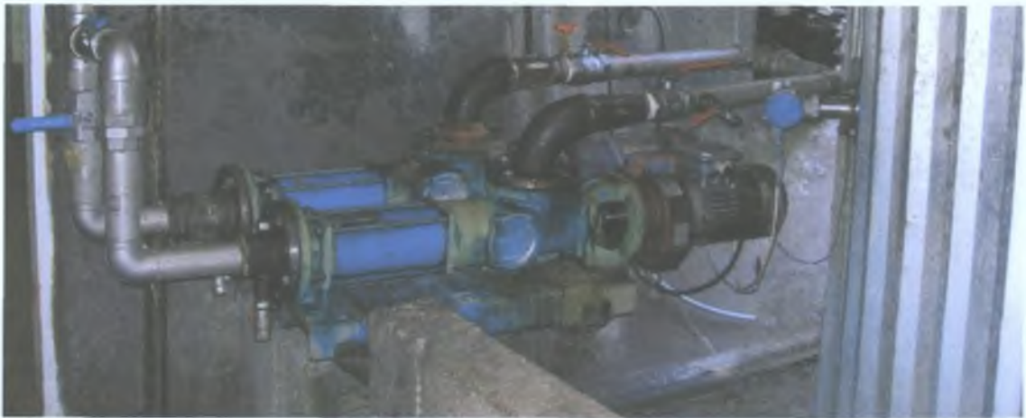
Plate 4.5.5 Pump and manifold used to pump tallow from the burn tank (on the right) around the tallow circuit.
