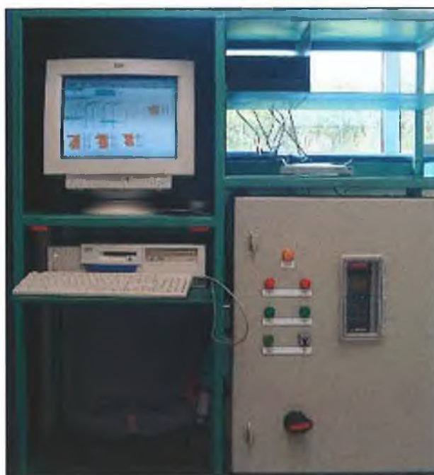
Figure 5.17 PC, NetDAQ and Inverter for Control of Compensation Fans
