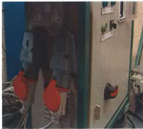
Figure 9A Shows Fan motor plugs connected on to the inverter.
