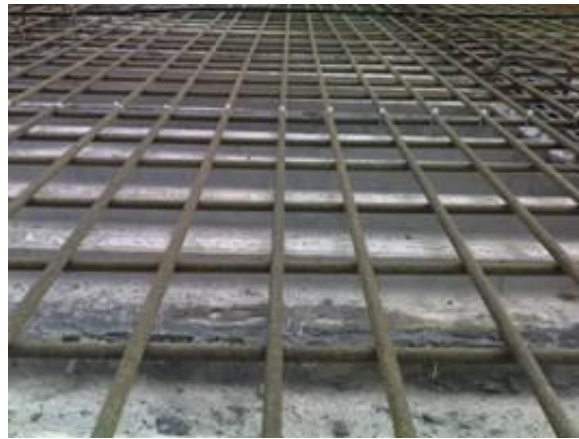
Figure 9: BFRP reinforced deck
