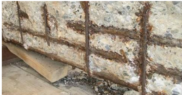
Figure 1: Chloride induced corrosion damage (Courtesy: http://cce.oregonstate.edu )
