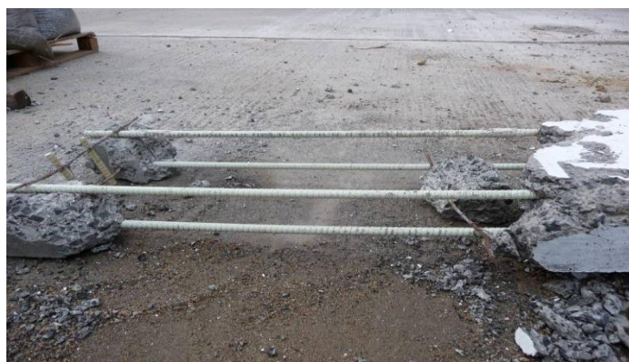
Figure 6: Condition of GFRP inside a tested slab (No indication of rupture on bars)
